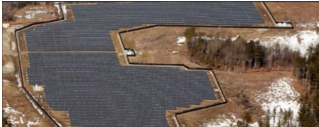
Aerial view of 3MW ground-mounted solar PV farm on the North Post.
