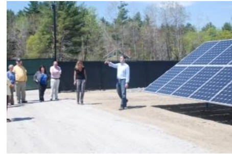
Brian Morrissey of Citizens Energy Corp. explains the design and development process for the installation of this 3MW solar photovoltaic panel farm on the North Post in Devens.
