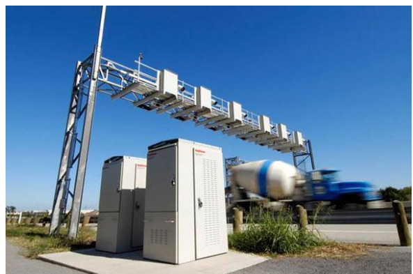
Example of high-speed electronic tolling gantry.
