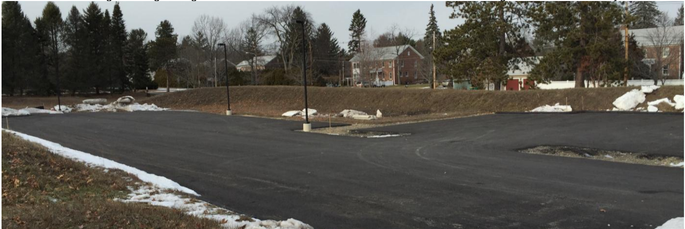
Laddawn parking lot expansion. Base course of pavement and light fixtures in place. Landscape berms also in place to provide visual screening from Jackson Road as well as adjacent residents.. Final landscaping, paving and striping to be completed in spring 2016.
