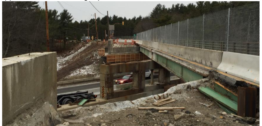
Jackson Road Bridge over Route 2 – looking south – Northbound lane of bridge decking removed. Southbound lane still open but only for access to south post – January 2016
