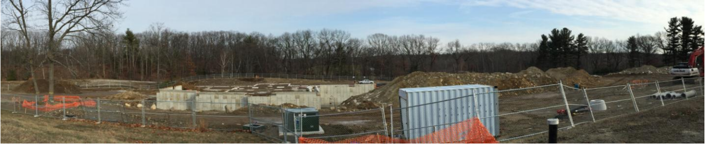
Looking east - view of Health Partners Treatment and Recovery Center building footings and westerly foundation walls – January 2016.
