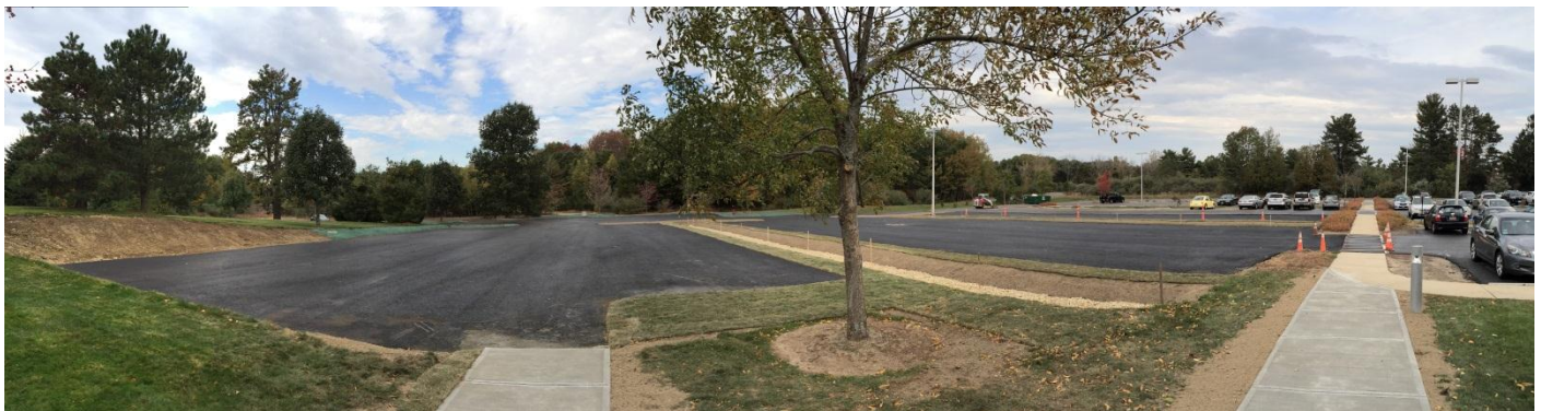
84 new parking spaces at 27 Jackson Road (biofiltration landscape islands installed without landscaping) December 2015.
