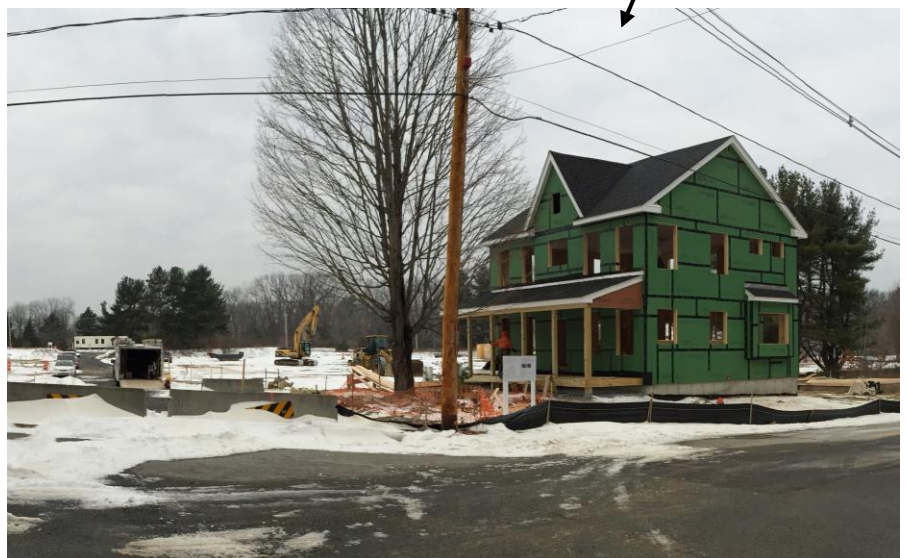
View of first new house at the Intersection of Chance and Antietam. January 2016
