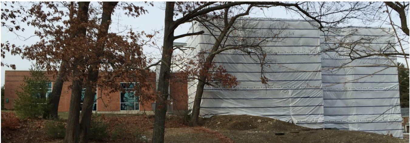
Side of Laddawn looking at existing building and new addition covered to allow for interior work to continue throughout the winter – January 2016
