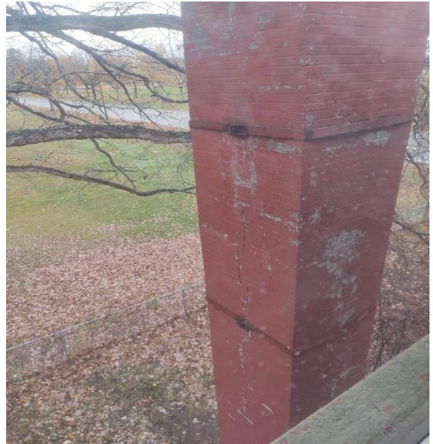
Image: Unbraced chimney, Washington Hall. (ICON Architecture, 2026.)
